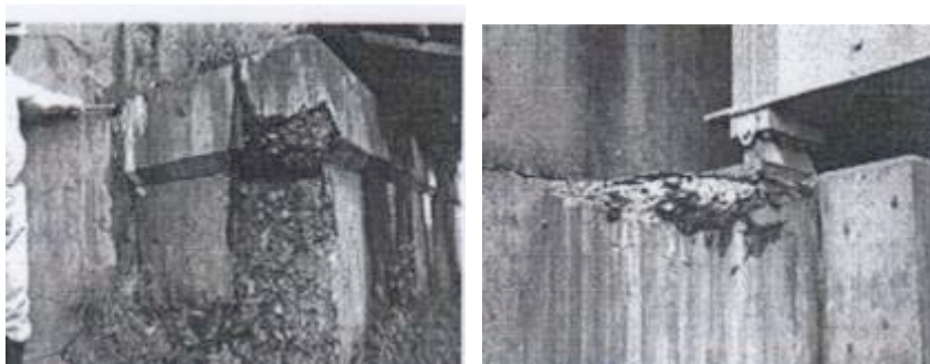
Figure 11. Damage due to freezing
