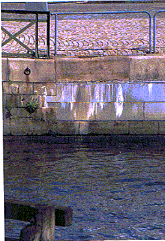
Figure 6. white precipitated salts, sticking hard over the blocks, Vallgrav, Goteborg.
