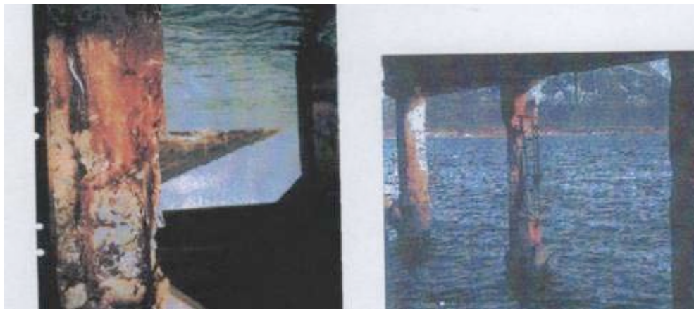
Figure 12 Photograph of pillar damaged by chlorides
