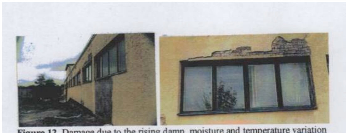
Figure 12. Damage due to the rising damp, moisture and temperature variation
