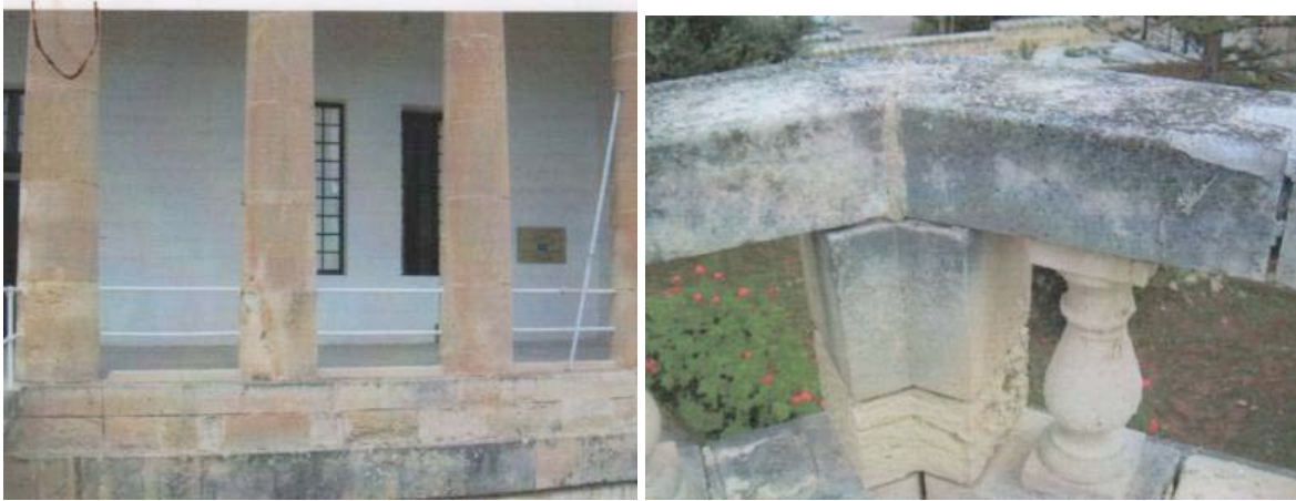
Figure 5. typical example of salt crystallisation, and acid rain, Malta (2007)
