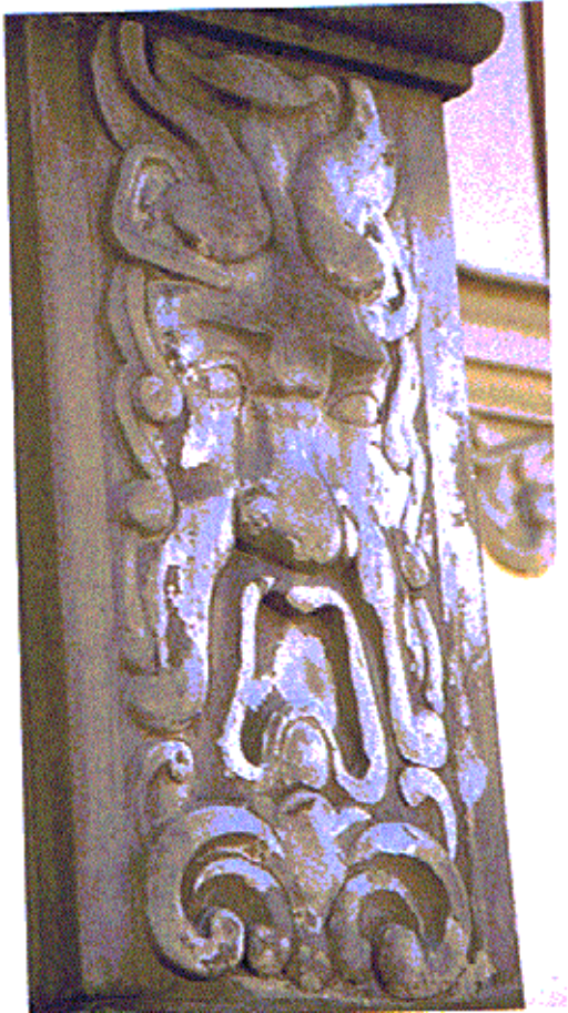
Figure 8. Deterioration after 20 years of exposure
